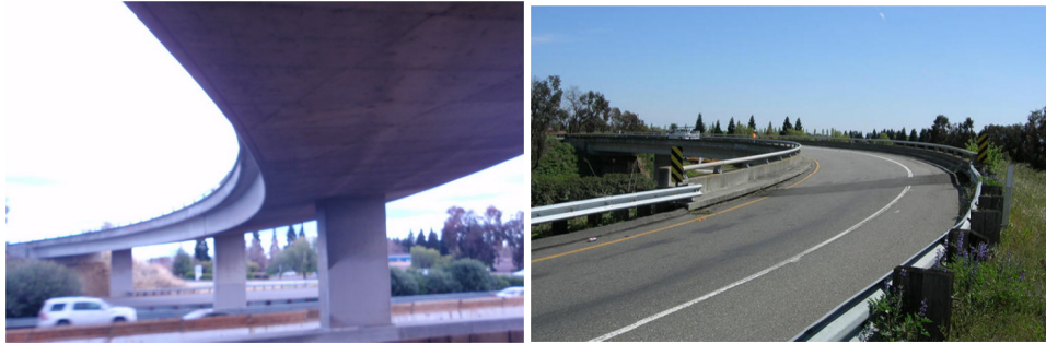
Figure 1. Under view of span 4 looking towards abutment 1 (on the left), and Roadway looking back on route (on the right) (source: Caltrans bridge inventory)
